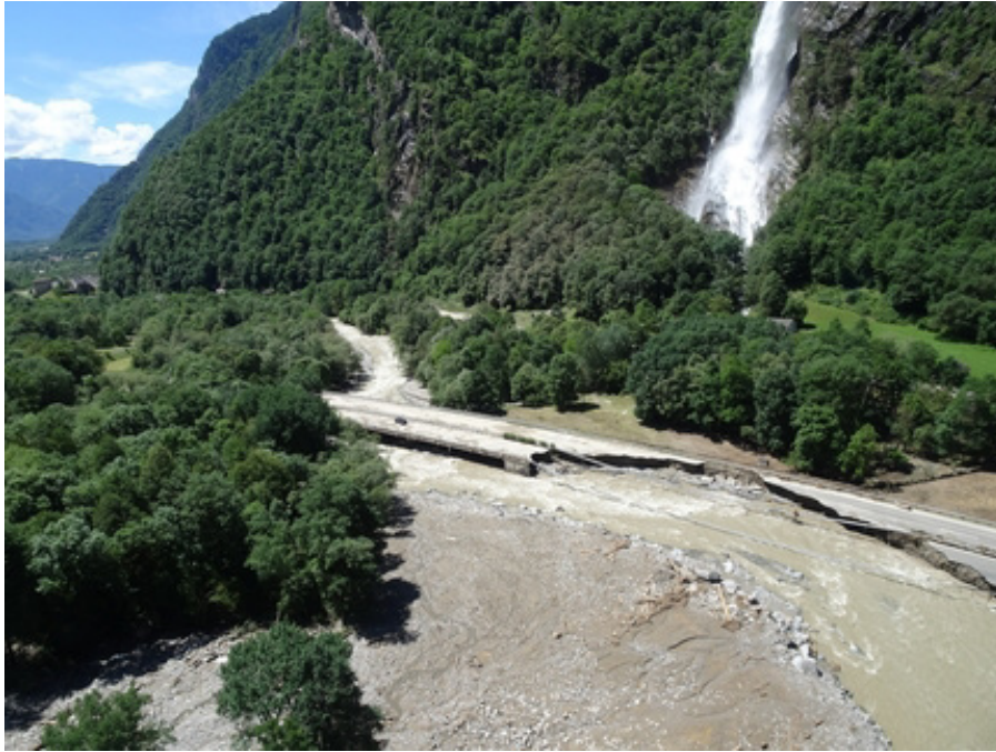
Bank erosion leading to significant infrastructure damage in Misox, Switzerland in 2024 (Image: Cantonal Police Grisonsr Zeitung)
