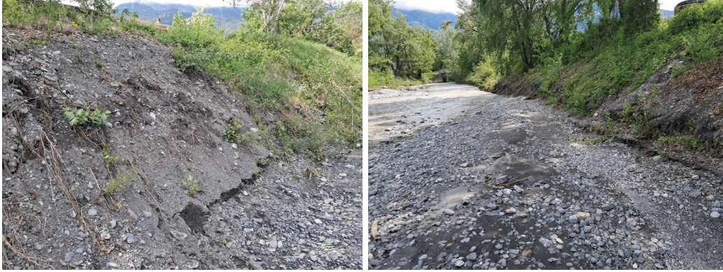
Figure 16: Pictures of the hydrographic right bank of the stream La Morge (downstream of the selected cross section).
